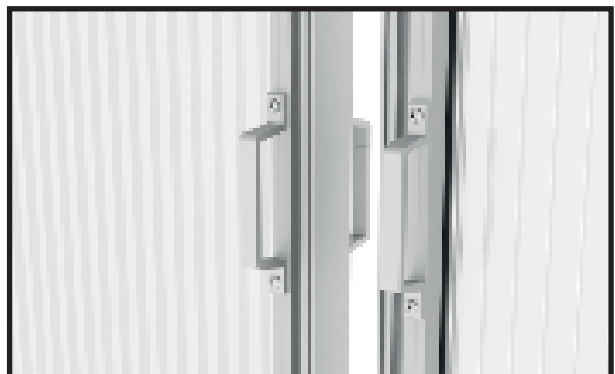
The installation of the door is completed after fixing the door handles inside and outside.
